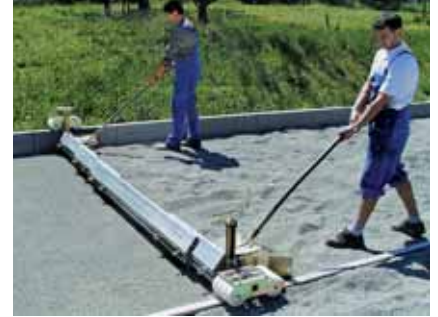
... screeding bedding material: all around good choice for large and small building sites – Telescopic Screeding System TAS-uni
